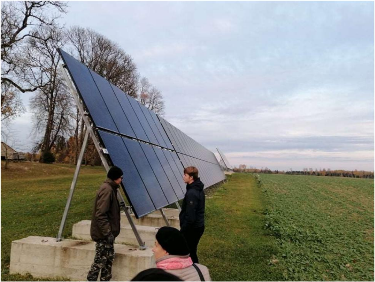
Solar panels in Clean Water theme park in Estonia (production of energy for personal use)
